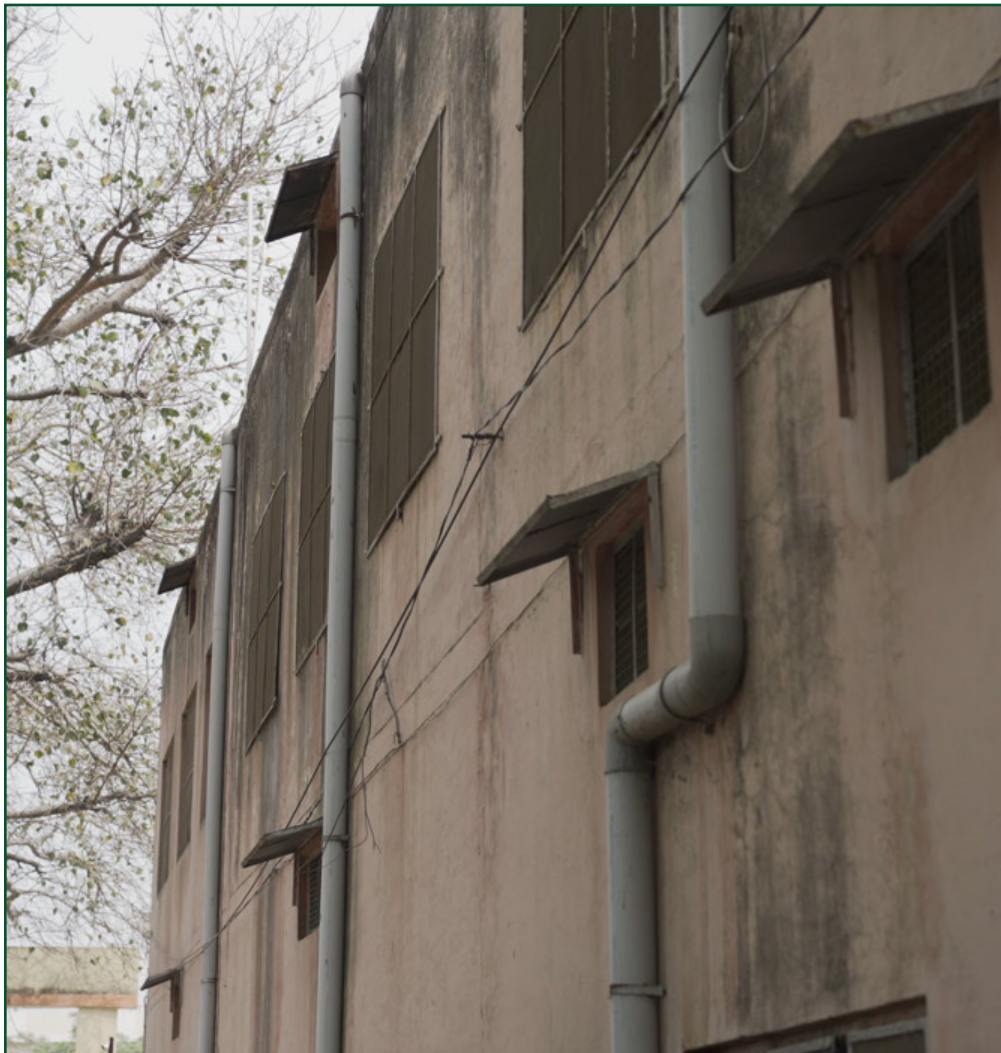
RWH Structure down pipe
