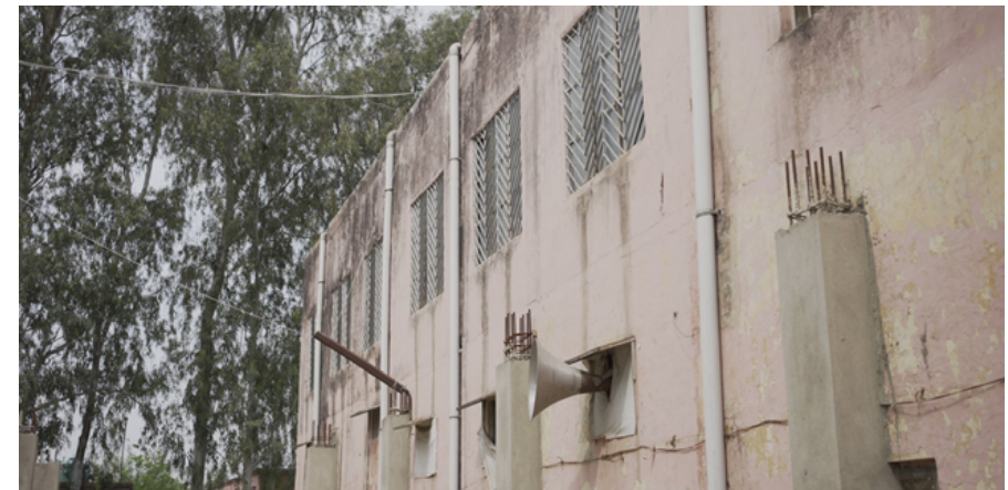
RWH structure downpipes
