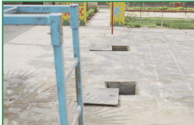
Desiltation chamber for RWH
